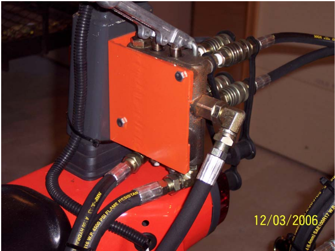
Picture 3 (Rear Remote lines)
